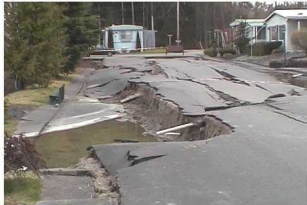
h) Collapsing soils, karst conditions, or liquefaction
