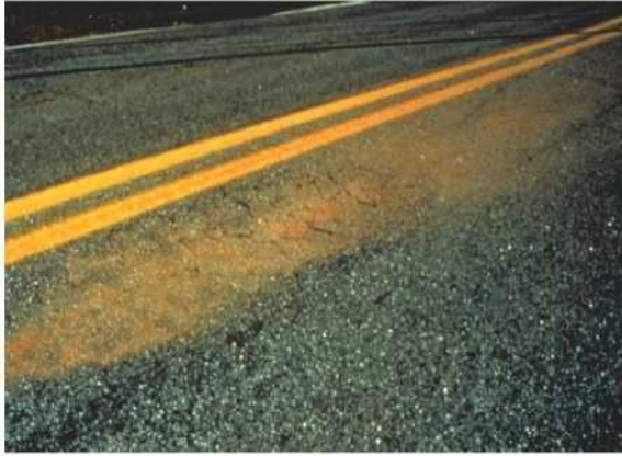
c) Subgrade pumping
