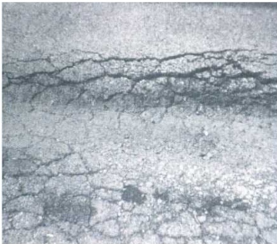
a) Excessive rutting
