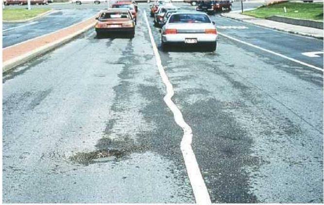
d) Drainage problems
